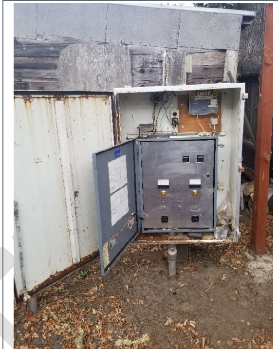
Photo 5 Lift Station 2 Cabinet
