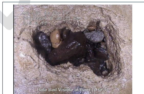
Photo 3. Hole/Broken with Voids Visible
